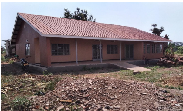
5. Nakigo CLC before being commissioning on 19th september 2023
